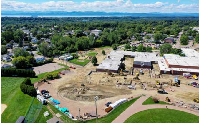
Looking west/southwest towards new Elementary addition. Excavation and concrete foundations are under way. In October, structural steel installation will begin.
